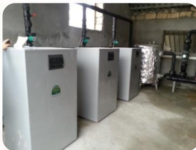
Secondary school № 149 (60 KW heating)
