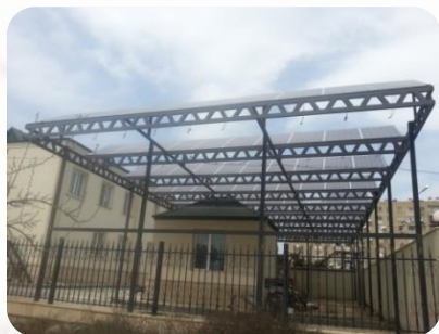
Pediatric Polyclinic (25 KW electric, 40 KW heating)
