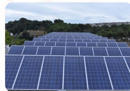
Secondary school № 235 (25KW electric, 40KW heating)
