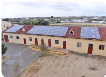
Boarding school in Turkan (25 KW electric)
